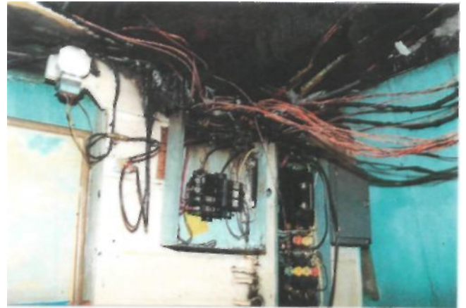
Figure - Over 25% of fires are caused by electrical
