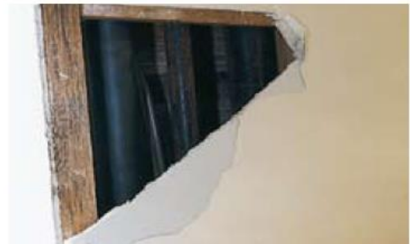
Asbestos insulating board (AIB)
